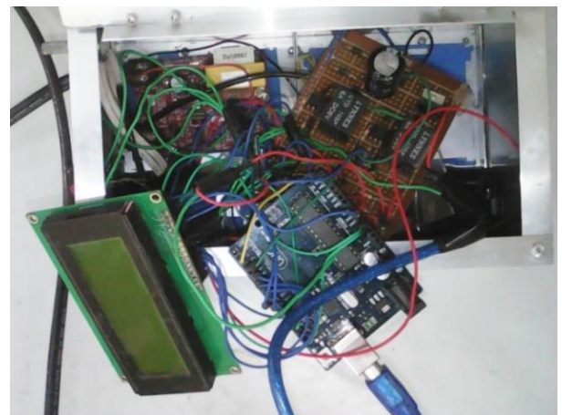
Figure 3: Power Factor Correction Device
